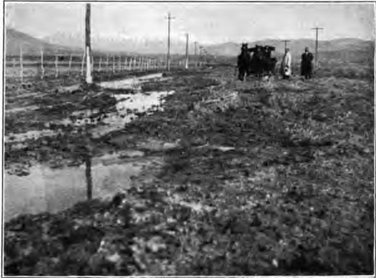
FIG. 9. LOOKING NORTH TOWARD FOUNTAIN GREEN. THE PICTURE SHOWS A PORTION OF THE STATE ROAD JUST BEFORE THE WORK OF CONSTRUCTION WAS BEGUN IN THE SUMMER OF 1910
